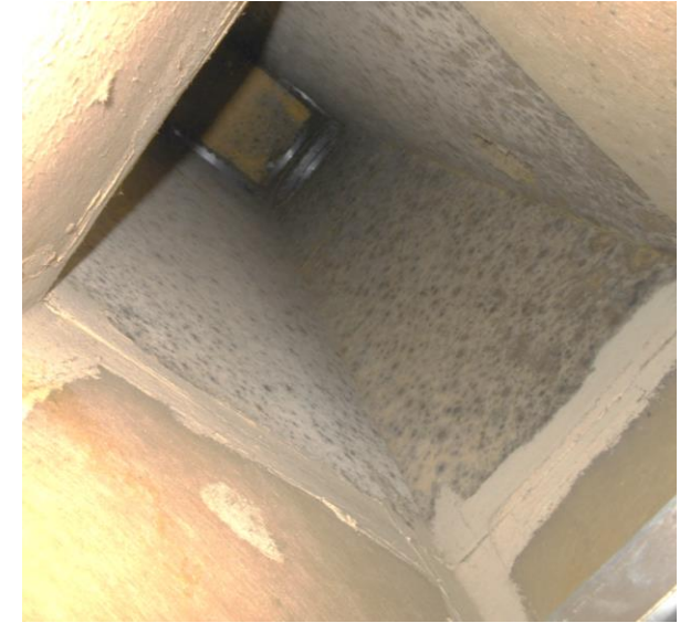
Mold growing on the lining of AC supply plenum.
