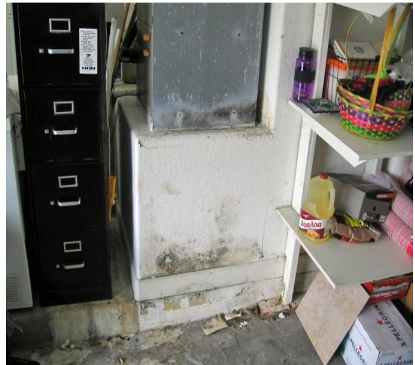
Water damaged AC return air box with mold both outside and inside
